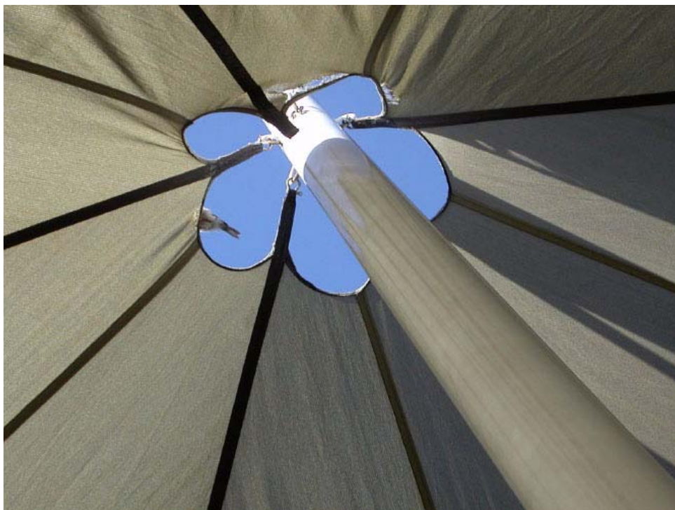
Figure 3 – Shadecloth structure at School, installed 2000, repaired 2006
