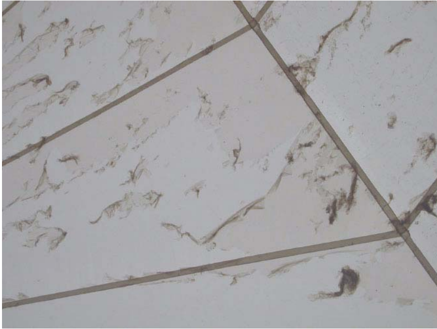
Figure 6 – delamination of surface coating on pvdf/pvc-coated polyester, installed 2000, coating issue arose at end of 2003
