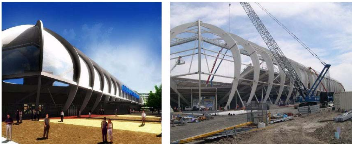
Figure 5. Presentation image on left showing stadium from South–East corner and construction photo taken in late September 2007.
