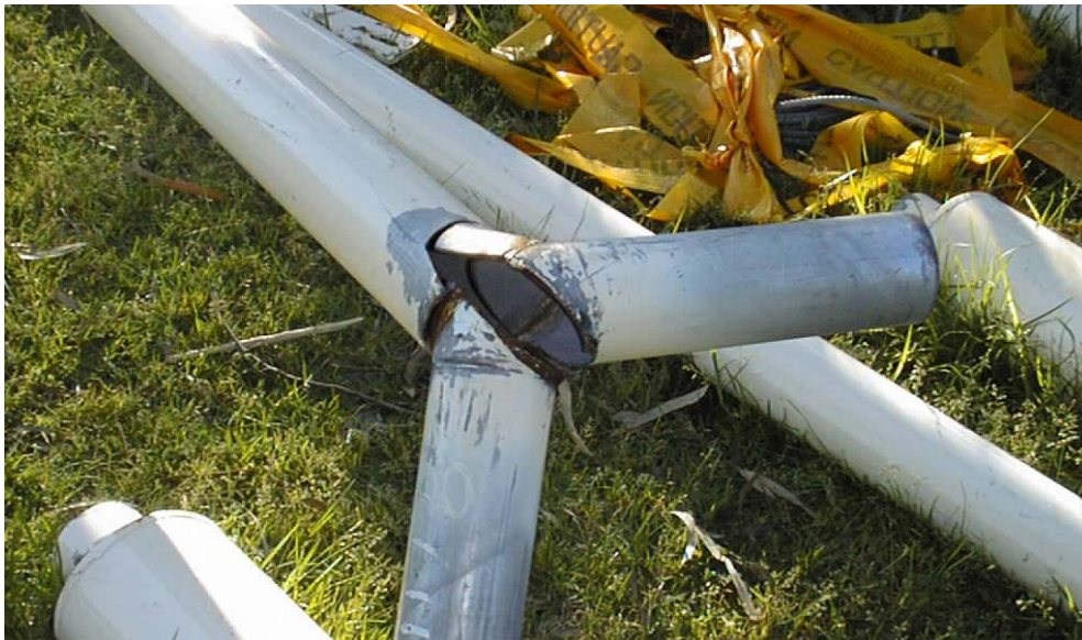
This hip and ridge “Y piece” has suffered sudden and catastrophic failure under wind load.
