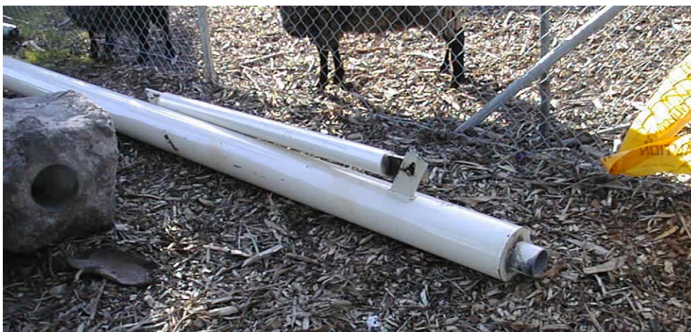
Note the shallow concrete footing to the left. This post and footing was completely lifted clear of the ground during failure. The original structure covered a large primary school playground area approximately 140m 2 .
