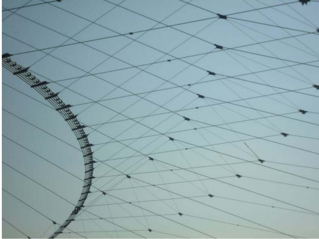
picture 17: Cable net of Durban
