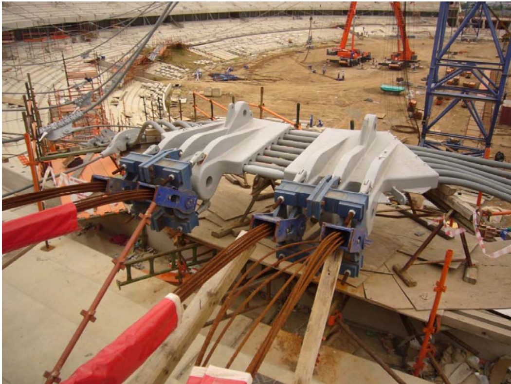
picture 14: Ring cable connector at tie backs
